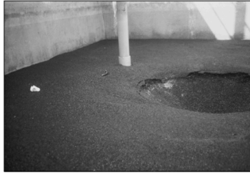
Source: John L. Cleasby, Filter Maintenance & Operations Guidance Manual . Figure 6-10 Cone of depression in filter media resulting from loss of nozzle in filter bottom
